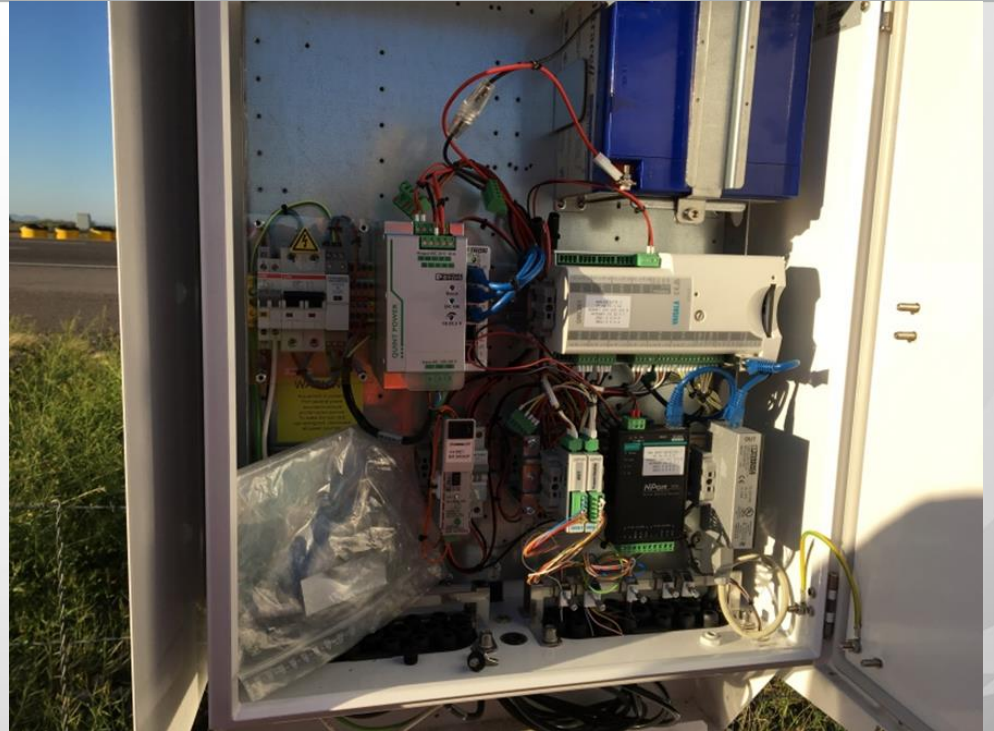
AWS310 (the brains) Each of the three locations talks to all 13 visibility sensors
